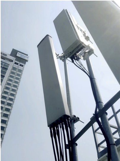
Figure 4: Co-located 32T32R and 8T8R MIMO antennas
